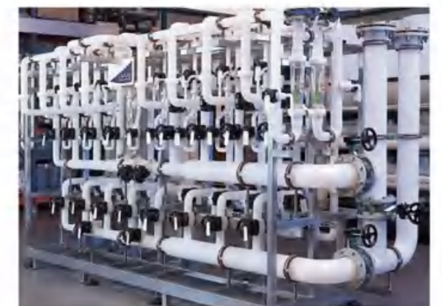
超纯水生产设备 Ultrapure water production equipment
